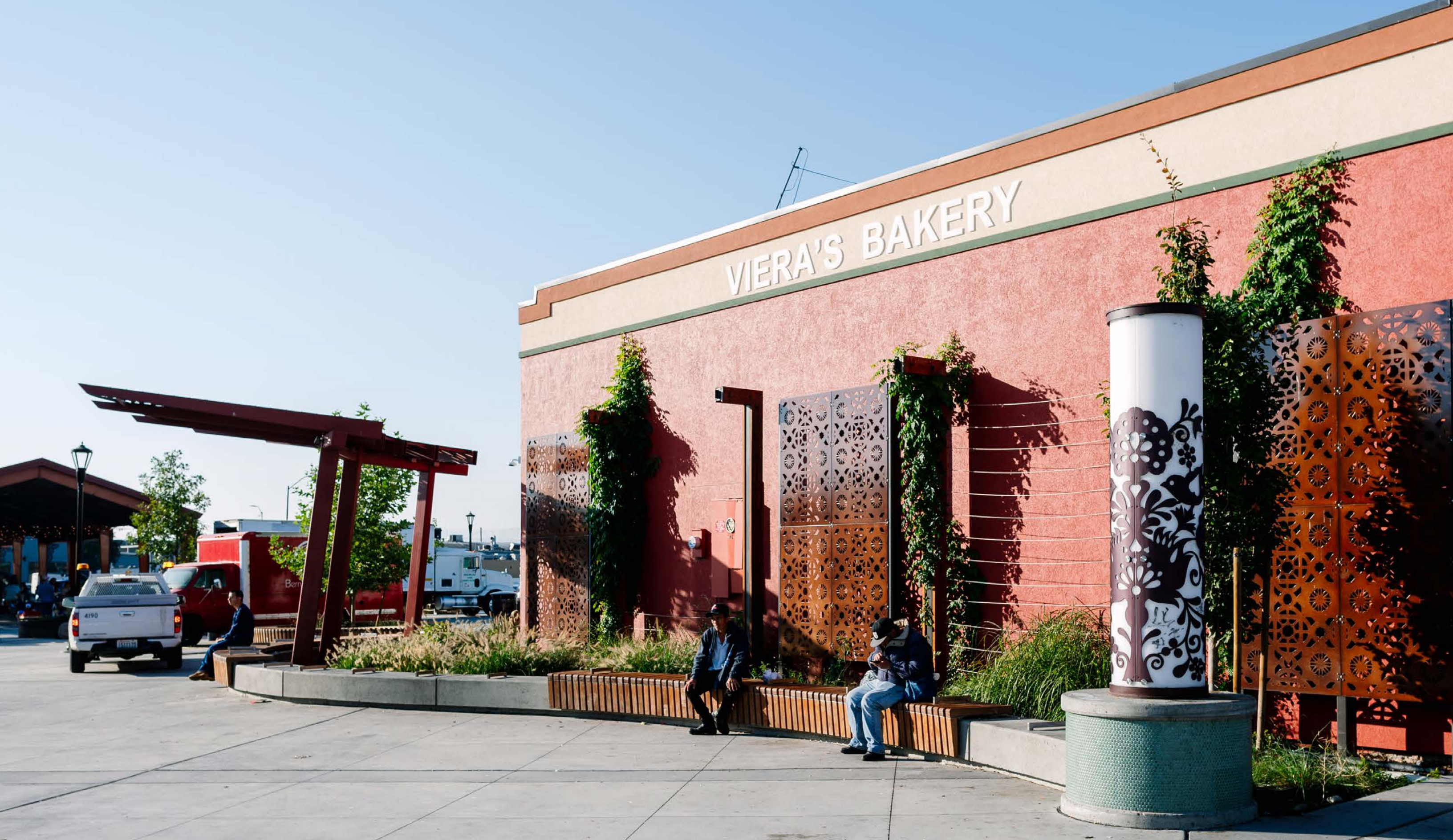
The City and design team worked closely with adjacent property owners to help ease impacts during construction. The team also coordinated with the businesses to provide facade repairs and improvements, including new stucco and paint, signage and screening.
