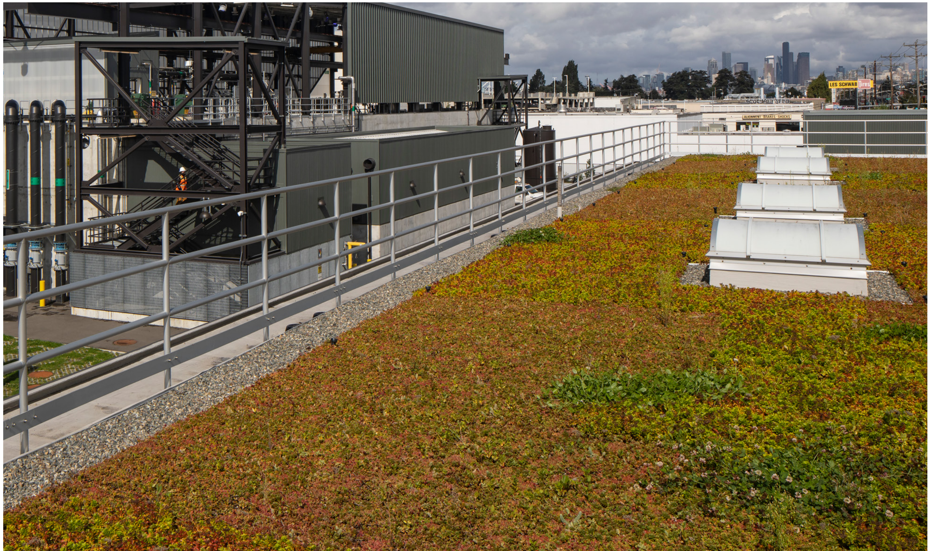
The vegetated roof atop the operations building adds an additional layer of GSI to demonstrate to school groups and the public how onsite stormwater is managed and how to reduce the heat island effect.
