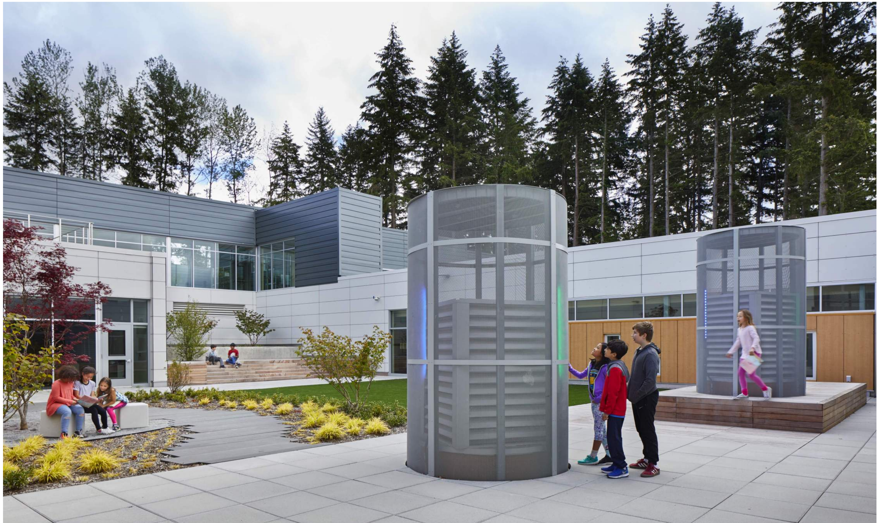
Large mechanical intake and outflow stacks are highlighted with decorative metal screens and LED light displays. Set amongst an ornamental landscape, the stacks become as much sculptural as they are functioning infrastructure.
